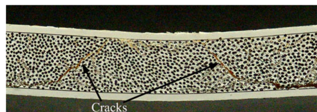
Fig. 13 A close view of the closed cracks of the panel without in-plane loading
